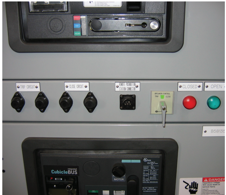
Control port on WL Switchgear
